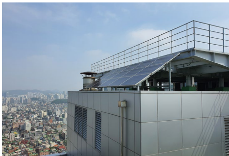
[Solar Power Generation Facility at KB Insurance Building in Hapjeong]
